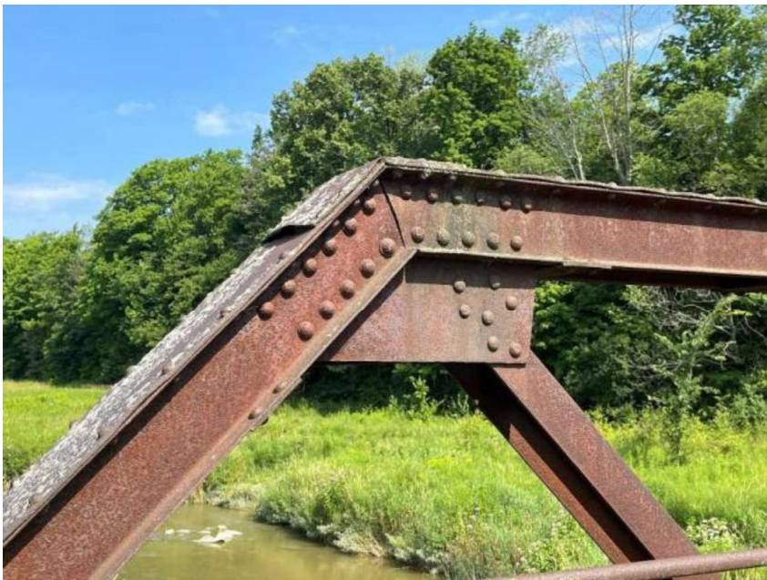
Figure 20: Detailed of riveted connection on west truss at the south portal, looking northwest (A.S.I., 2024)
