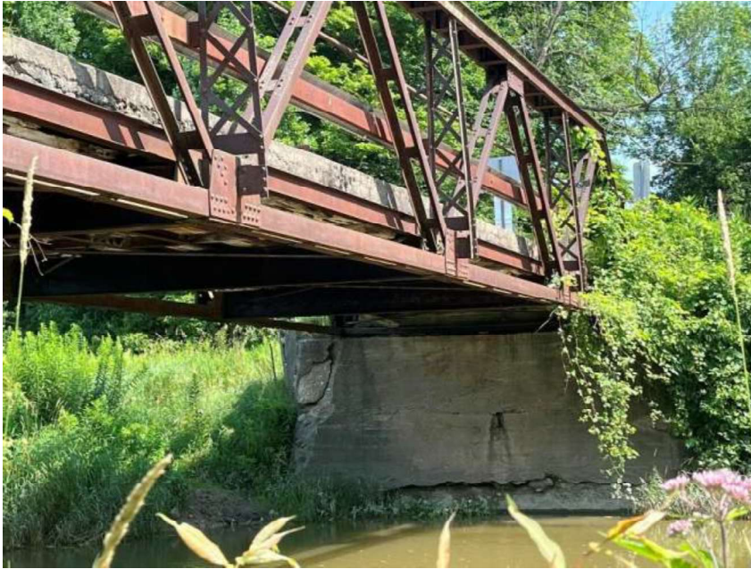
Figure 13: North abutment, looking north from the bank southwest of the bridge (A.S.I., 2024)
