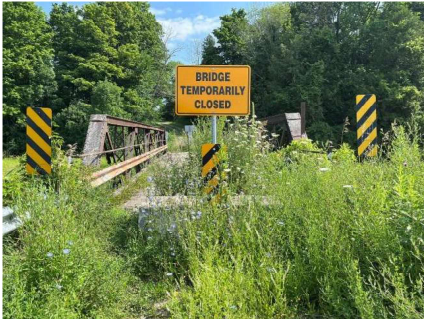
Figure 21: Bridge closure sign and concrete barrier at south approach, looking north (A.S.I., 2024)
