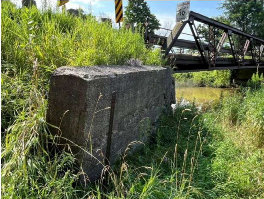
Figure 15: Angled wingwall on the northwest quadrant, looking southeast. Note the wooden board formwork impressions in the concrete (A.S.I., 2024)
