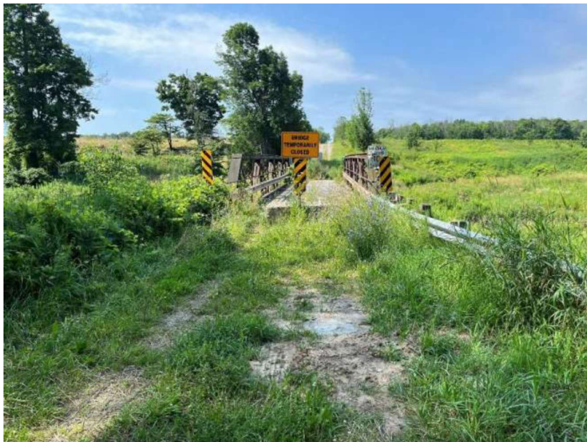
Figure 22: Bridge closure sign and concrete barrier at north approach, looking south (A.S.I., 2024)
